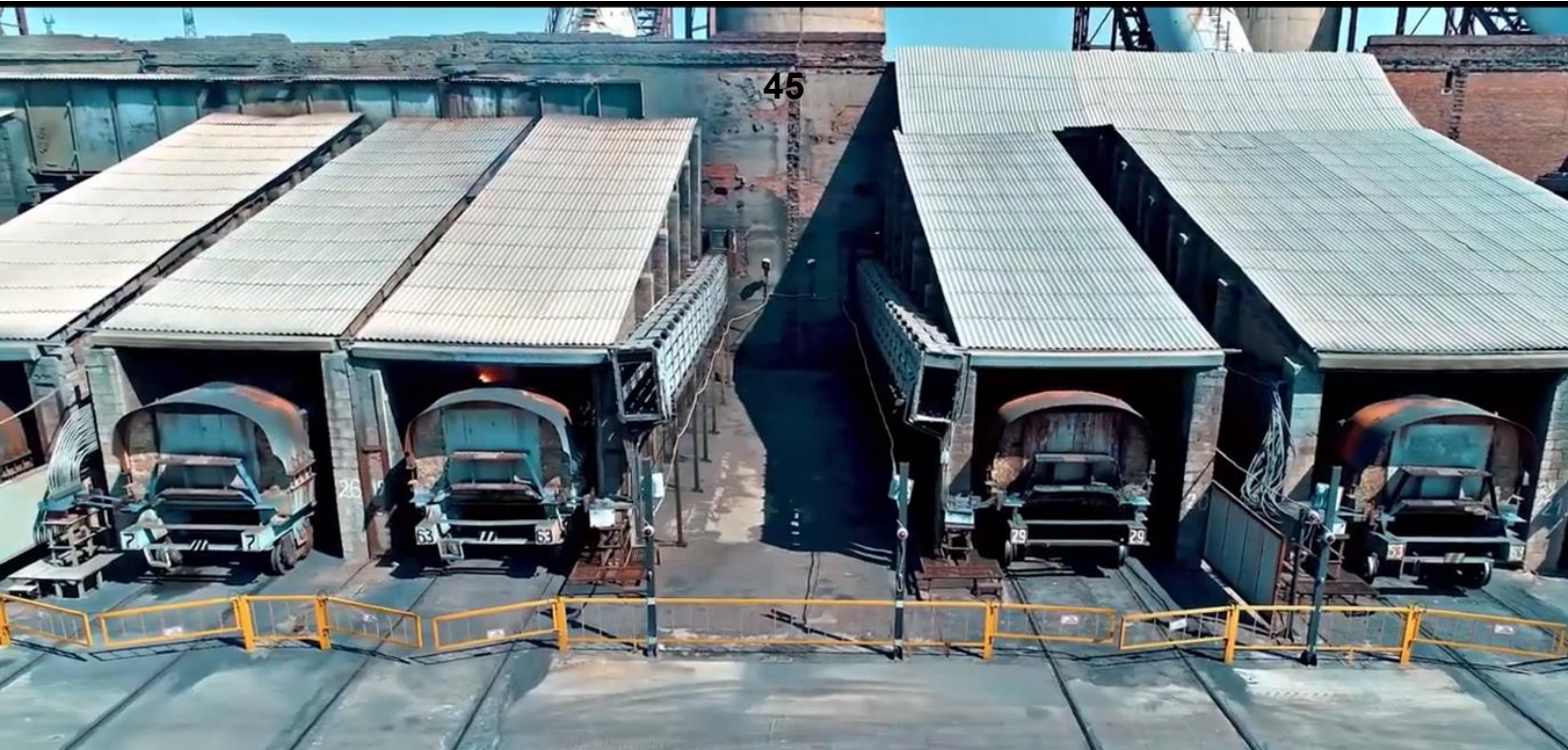
The furnace with hood system
